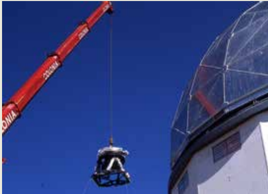
The lift of the hexapod after the installation of the tracker beam
