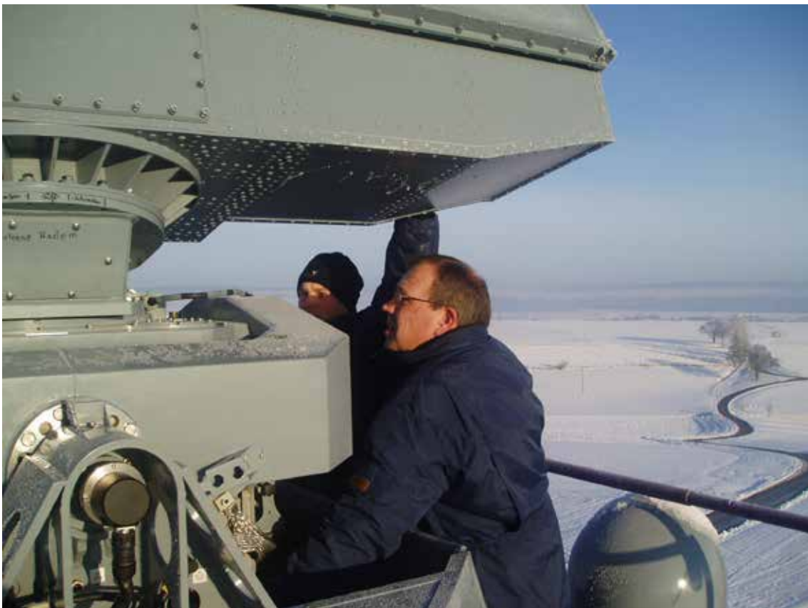
Installation against a snowy background of the stabilised platform developed for EADS in Germany
